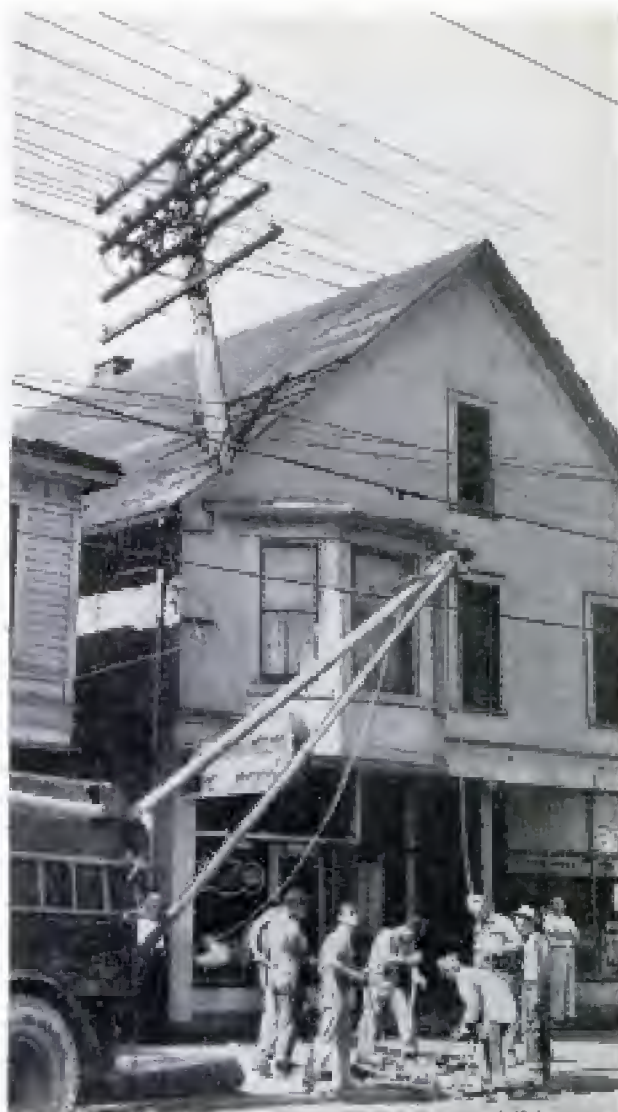
Cleveland Electric Illuminating Co. photo Electric pole stuck into roof top by tornado posed problem for Cleveland crew. Some wires remained hot
